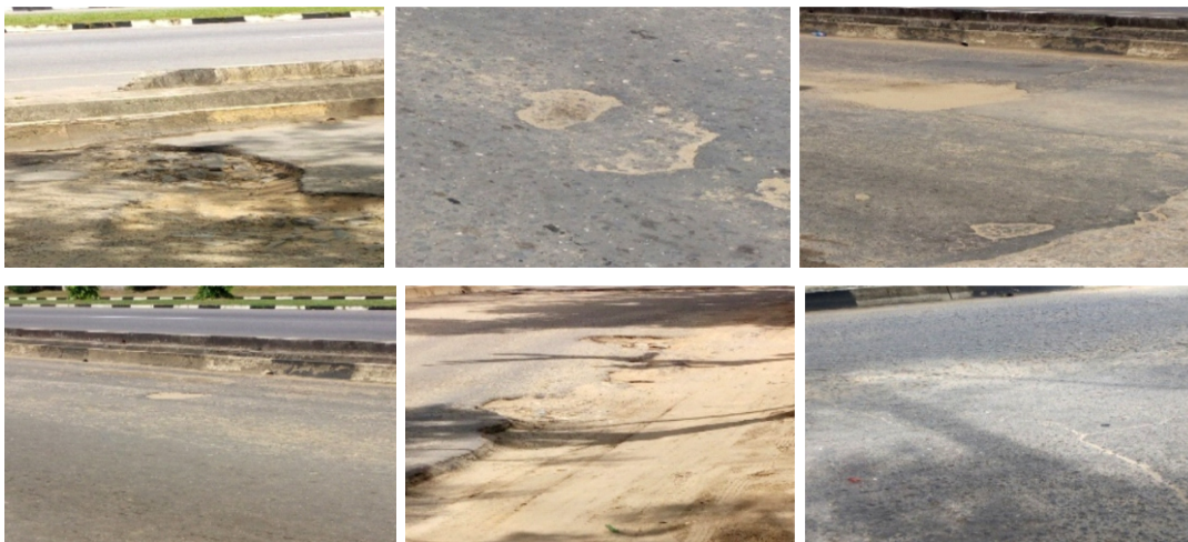
Fig. 2: Various failed sections of Edet Akpan Avenue
